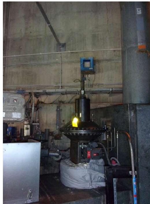
Fluorescent tag on steam dump valve
