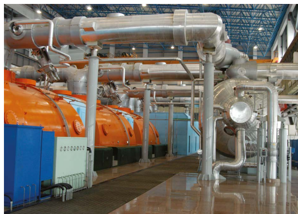
Turbine hall of Qinshan Nuclear Power Plant Phase 2 in China, June 2004. (Photo: P. Pavlicek/IAEA)
