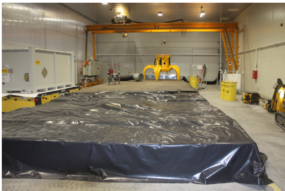
FIG. C.2. Infrastructure for decommissioning the RADON-type storage facility at Maišiagala, Lithuania. (Source: Ignalina NPP)
