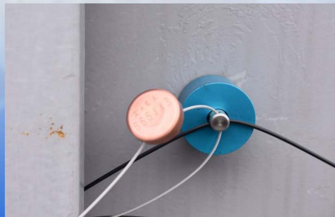
ISF-2贮存设施原子能机构封记完整
